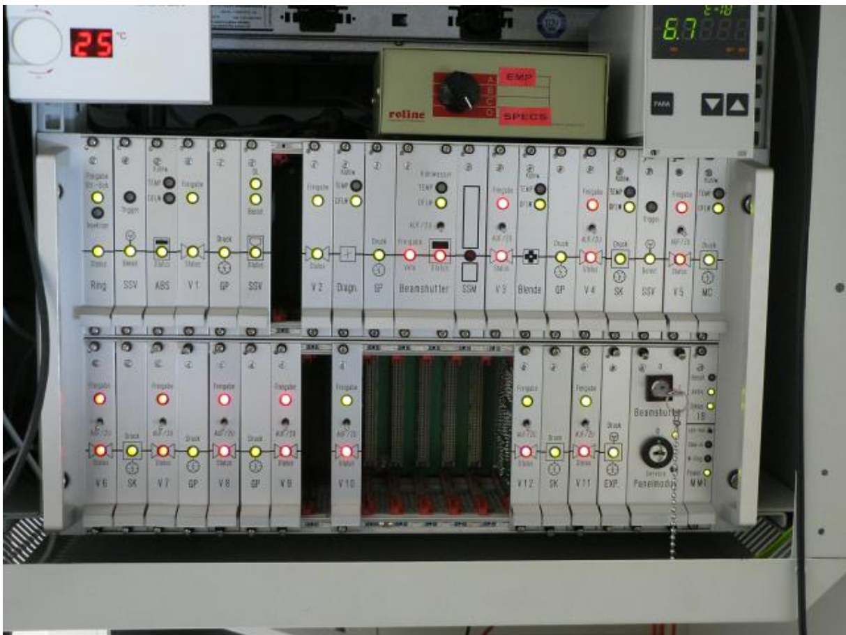
Figure 1: beam valve control panel with "roline" control box (to switch between XPS and NEXAFS); in the upper right corner you see the pressure reading of the beamline part just behind valve 13 on the beamline side.
