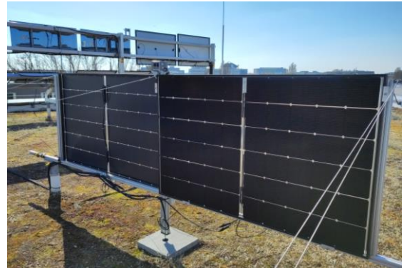
Fig. 2: Picture of the installation of the bifacial modules facing east and west, respectively with the optimized side. The bifacial modules were taken off the open rack and installed as shown here in December 2023.
