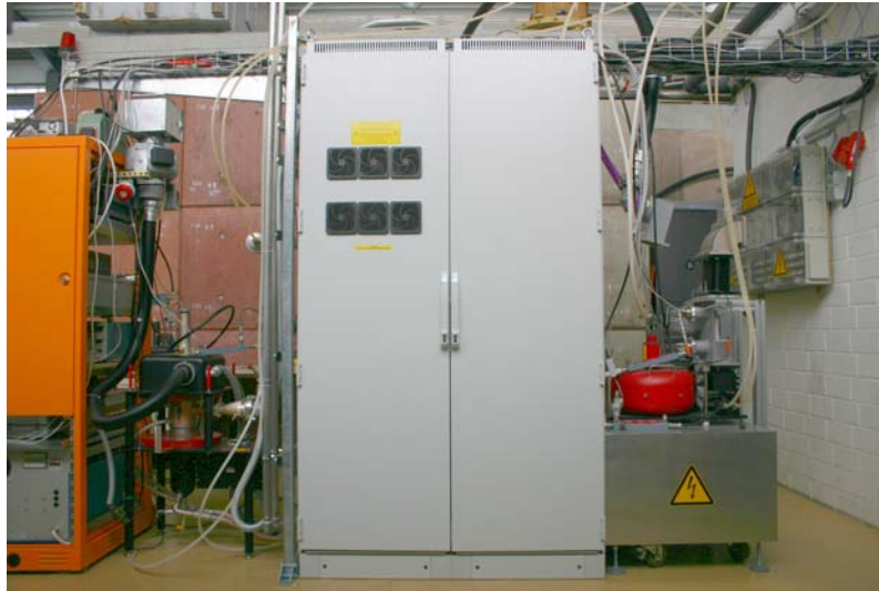
Figure 5.6: First HoBiCaT transmitter prototype: in the middle the power supply, right side the 10 kW klystron and left side an IOT prototype.
