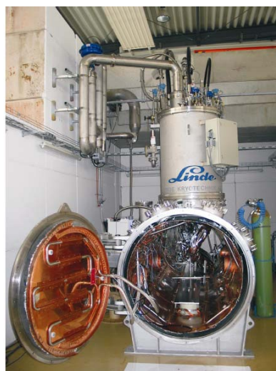
Figure 5.2: The BESSY Horizontal Bi-Cavity Test-facility (HoBiCaT).
